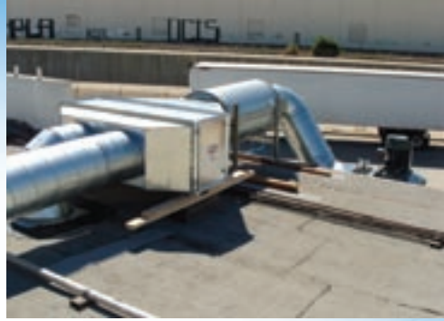
Exhaust duct from the SFC downward flow dust collector with in-line silencer and safety filter.
